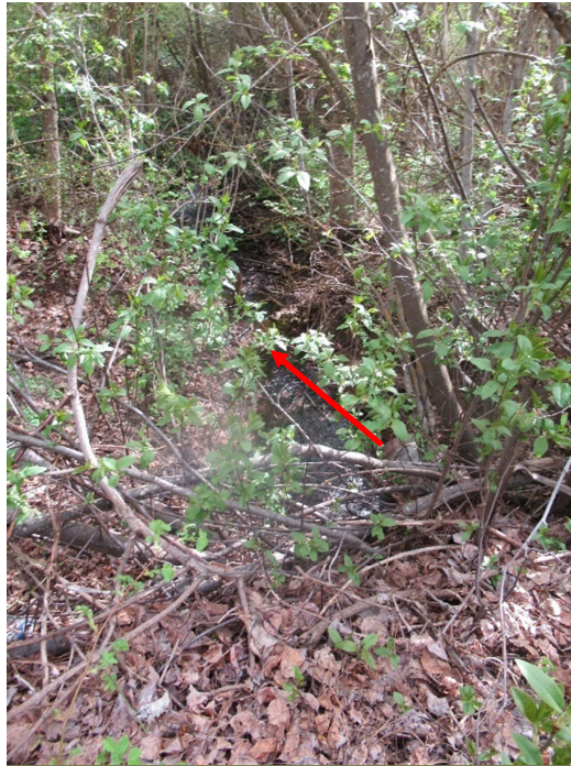
Photo 5– Facing southwest. Runoff flows out of 18" RCP culvert to flat bottom creek, heavily vegetated.
