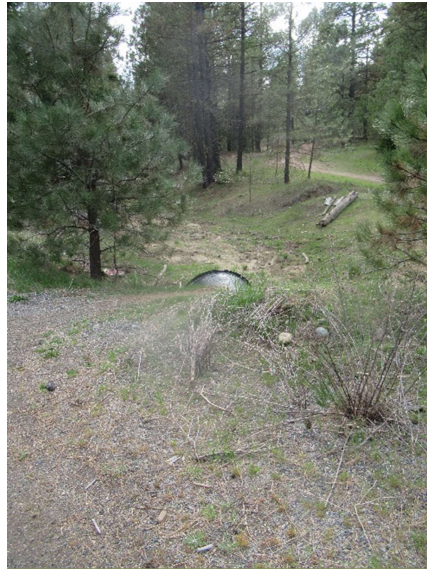
Photo 3 – Facing southwest. West of Summit View Drive. Runoff flows out of 48" HDPE culvert (Crystal Creek 3 Basin 3).
