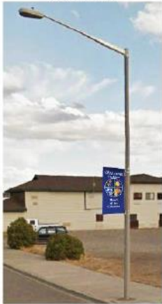
EXISTING STREET LIGHT With banner
