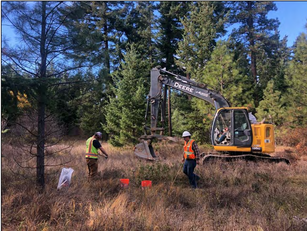
Figure 2. Overview of the typical conditions at geotechnical trench location EP-47, view to the west.
