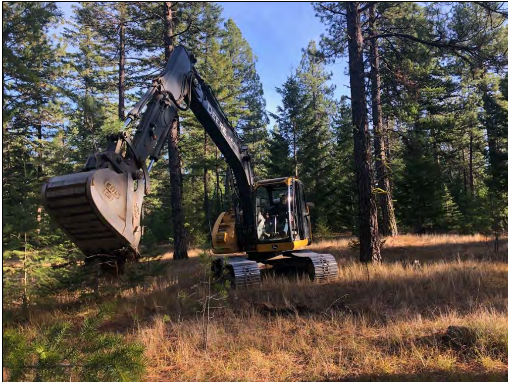
Figure 2. Overview of the typical conditions at geotechnical trench location EP-39, view to the southeast.
