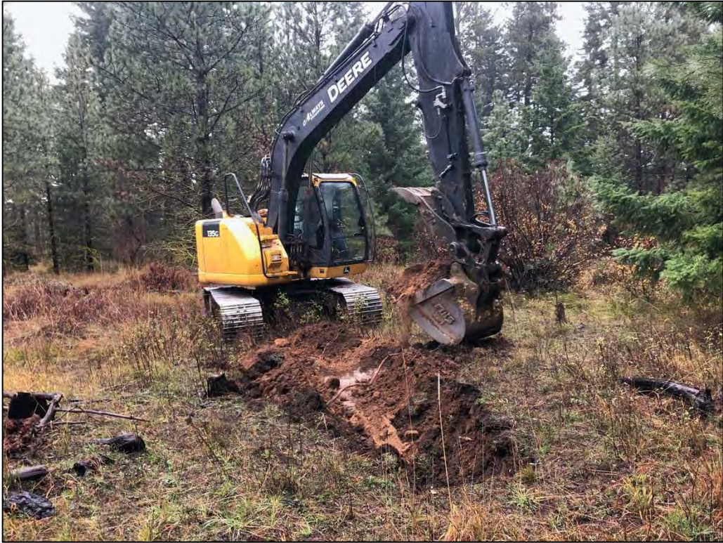
Figure 2. Overview of the typical conditions in geotechnical trench location as observed in EP-4, view to the north.
