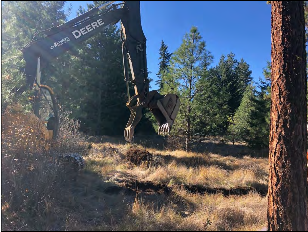
Figure 1. Overview of the typical conditions at geotechnical trench location EP-45, view to the southwest.
