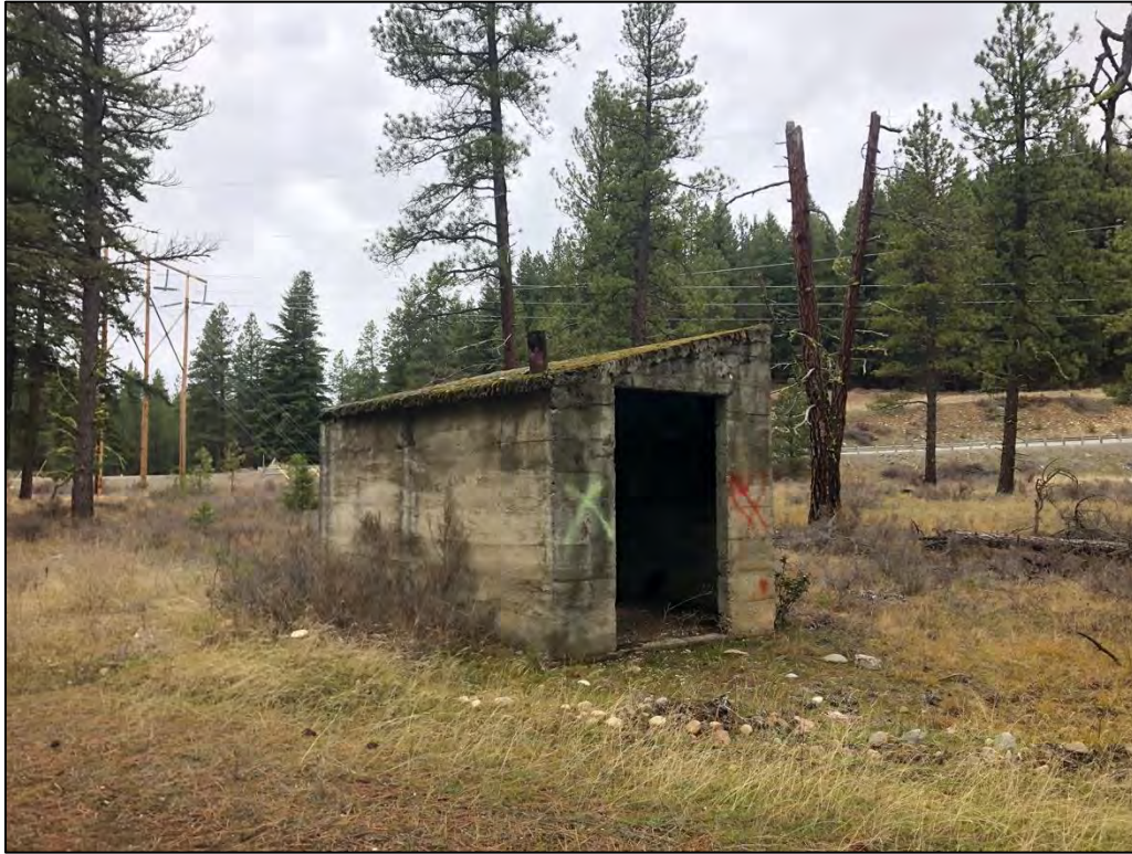
Figure 17. Overview of the chlorination building (45KT3331) associated with the Cle Elum waterline, view to the northwest.
