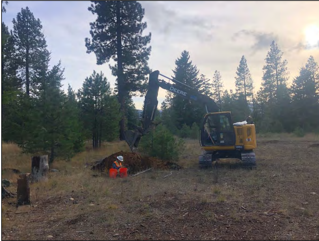
Figure 2. Overview of the typical conditions at geotechnical trench location EP-28, view to the south.
