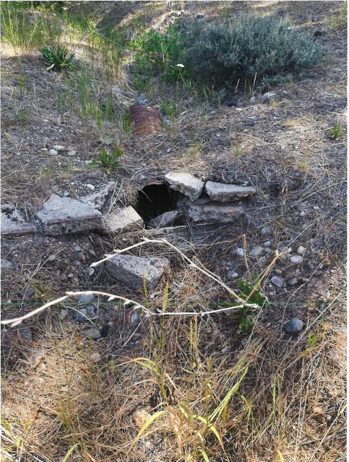
Photograph 5: Drainage on east side of parcel looking downstream, or the upstream of culvert.
