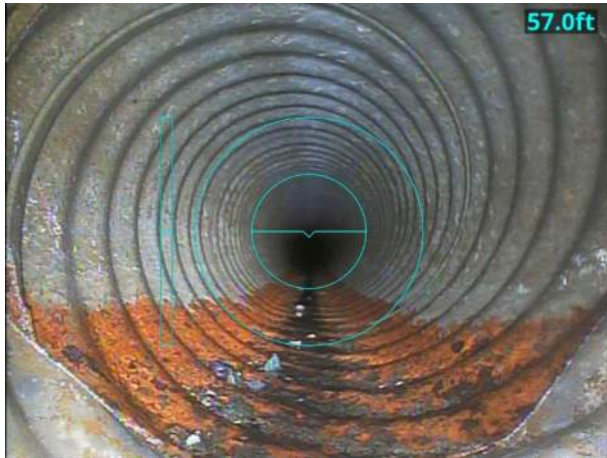
./3RD---COLUMBIA-NORTH-PT.2_2025_09_04-11_24_58_741.jpg 57.0 (ft) RUSTED PIPE
