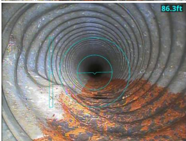
./3RD---COLUMBIA-NORTH-PT.2_2025_09_04-11_26_23_387.jpg 86.3 (ft) DENTED PIPE
